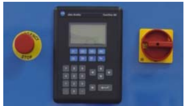
Master Control Panel Operator Interface
