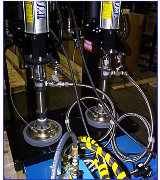
5-Gallon Part A and -B Supply Pumps
